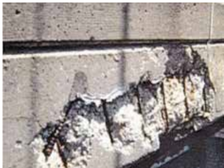
Figure 2. Concrete spall with exposed reinforcing bars and delaminated loose concrete at slab edge.
