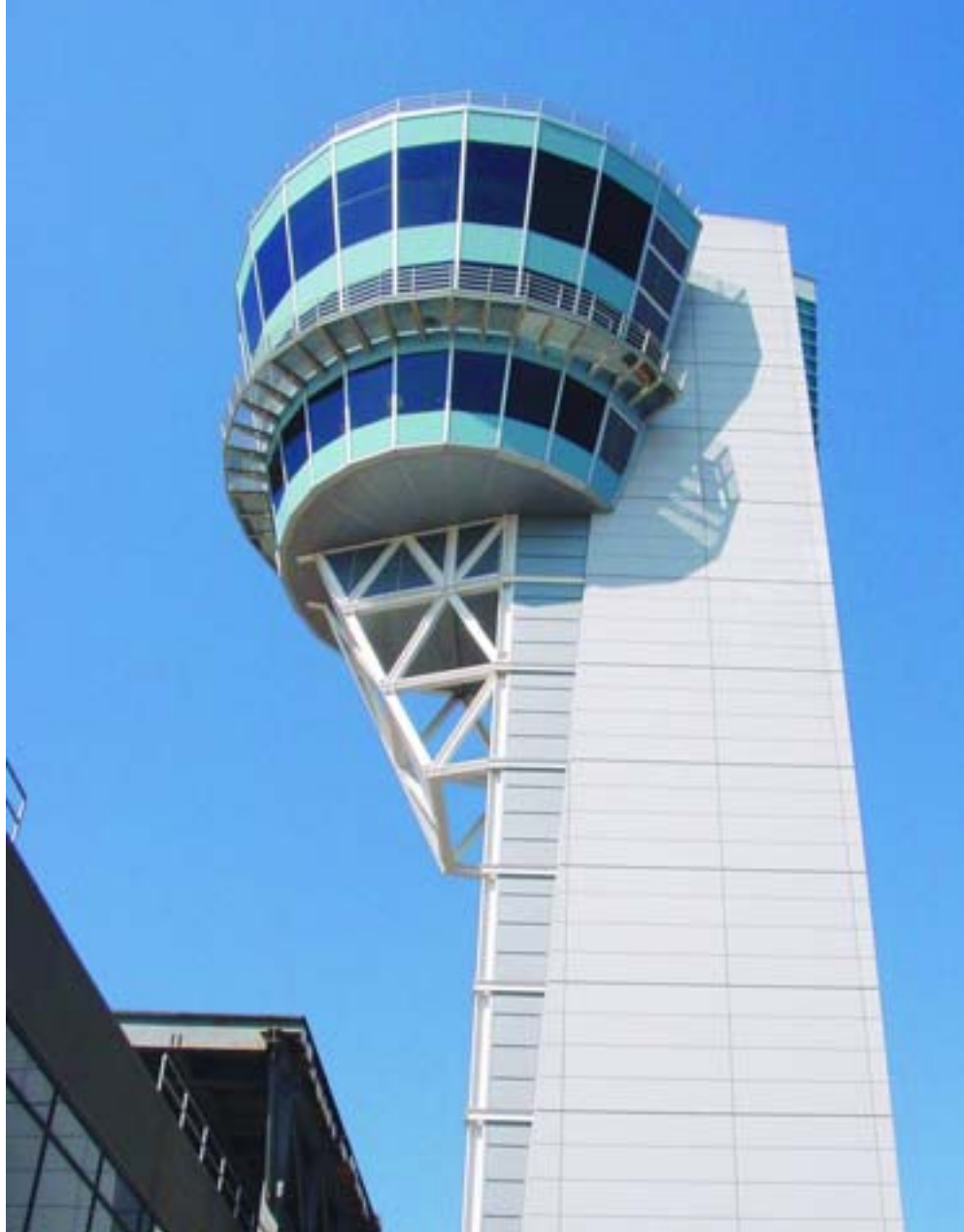
An intumescent coating protects the cantilever truss members against corrosion and fire while providing a smooth appearance.
